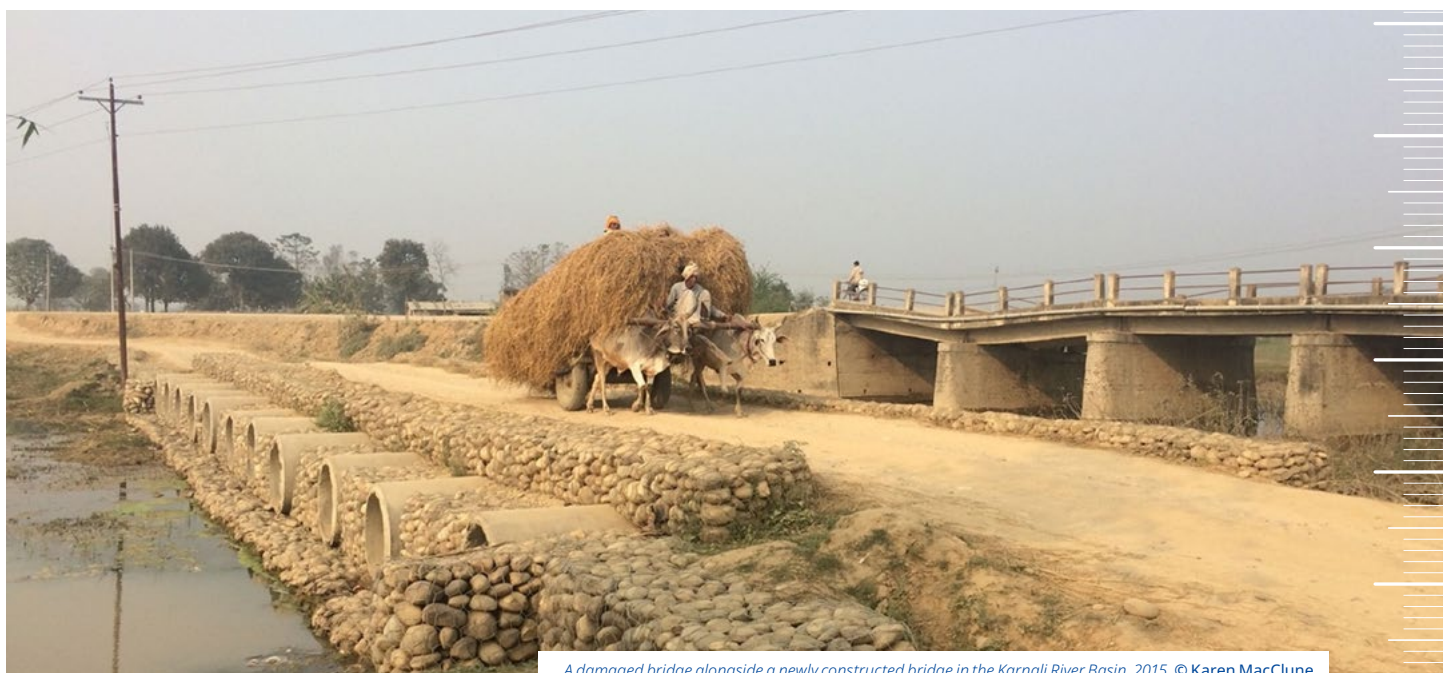
A damaged bridge alongside a newly constructed bridge in the Karnali River Basin, 2015. © Karen MacClune
