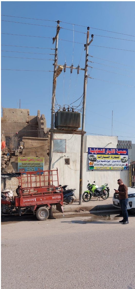
No circuit breakers
