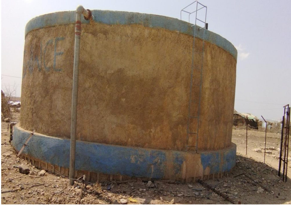
Figure 4-5 Existing 200m 3 service reservoir
