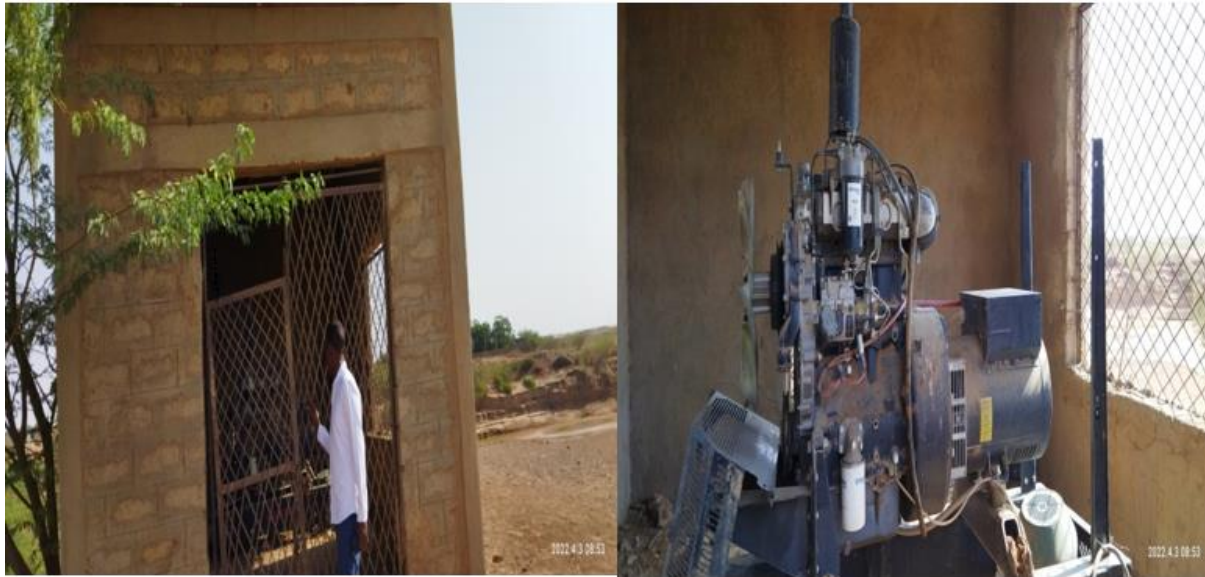
Figure 4-9 Pump station at river diversion and generator
