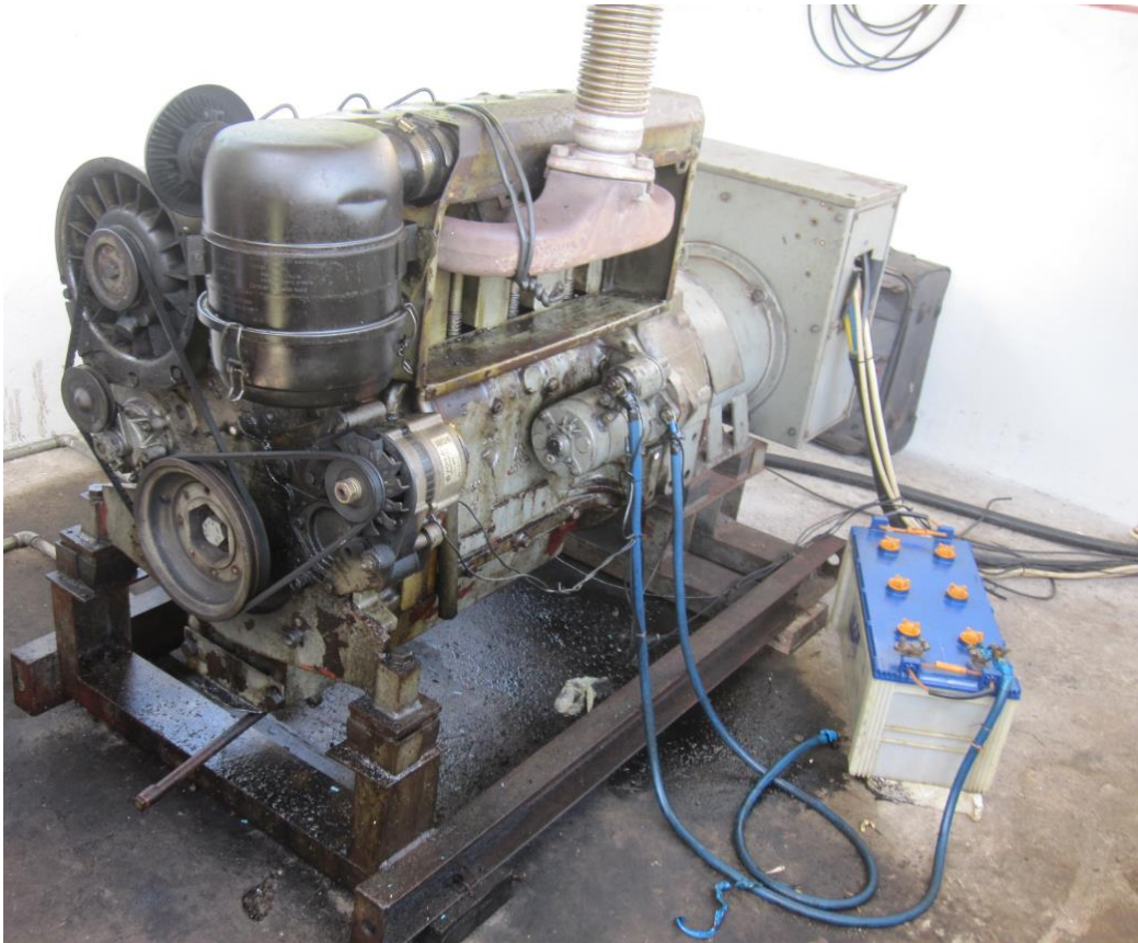
Figure 1: Existing Diesel Generator in P. Tiga site
