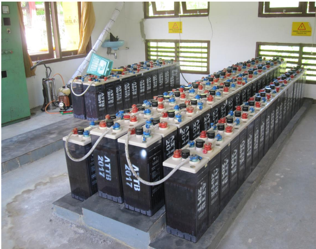
Figure 1: Existing defunct Lead-acid battery in P. Tiga site
