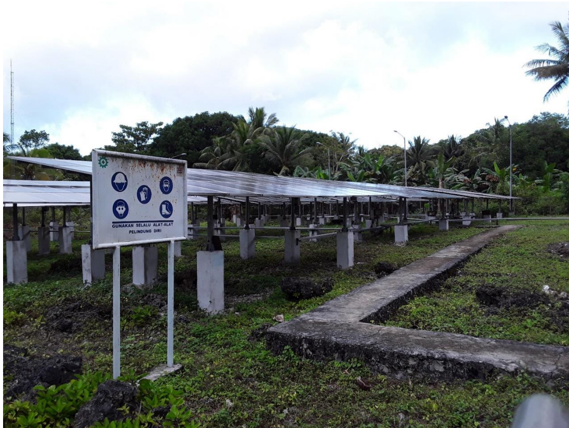
Figure 1: Existing defunct PV modules in P. Tiga site
