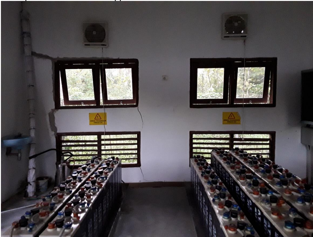
Figure 2: Existing Battery Room
