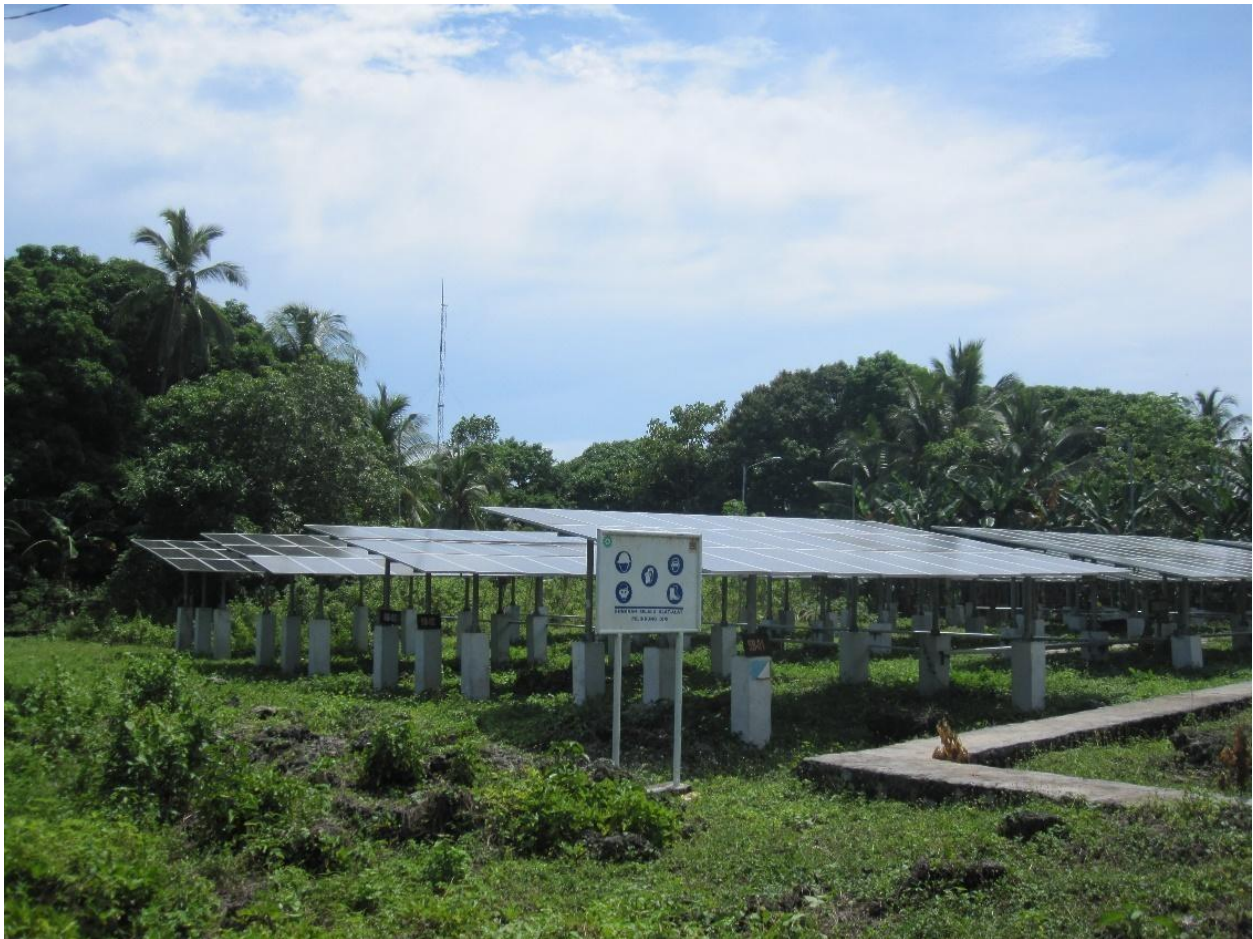
Figure 1: Existing un-operational solar-battery power plant PV arrays
