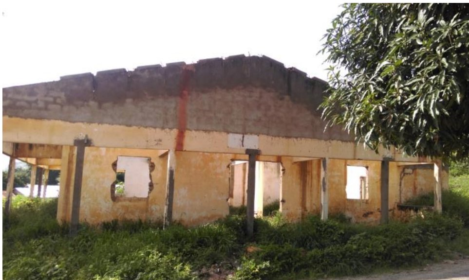
Infrastructure destroyed during the conflict in the Mamadou-Sara neighborhood (Credit: Thierry Vircoulon, Bouar, July 31 2017)
