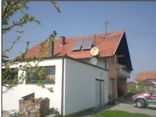
New solar systems installed on a home.
