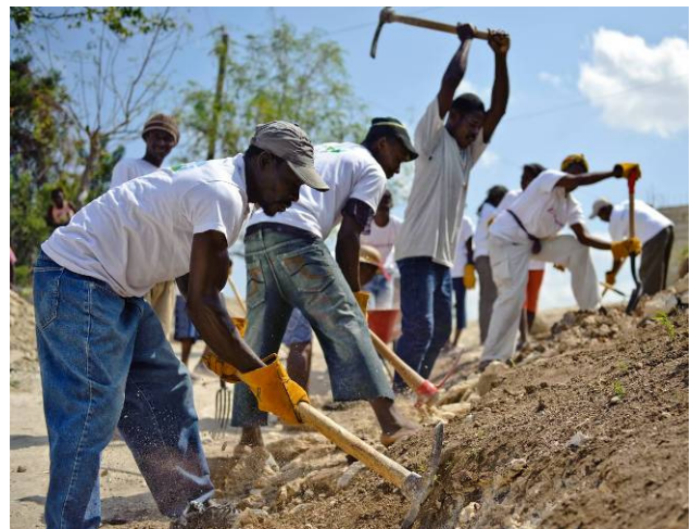
Our cash-for-work program is paying survivors a fair daily wage to clean and repair earthquake damage, putting cash back in households and local economies. Photo: Miguel Samper for Mercy Corps
